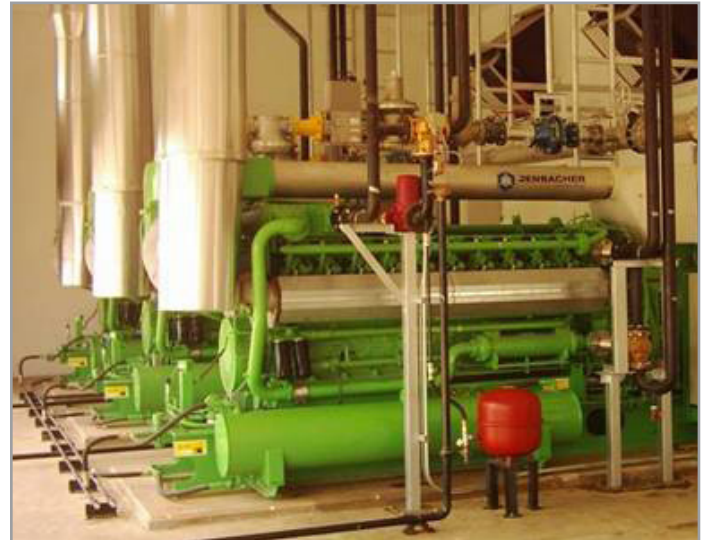
The methane is then burned in three 1 megawatt generators to make electricity. Photo courtesy of Palang Thai.
